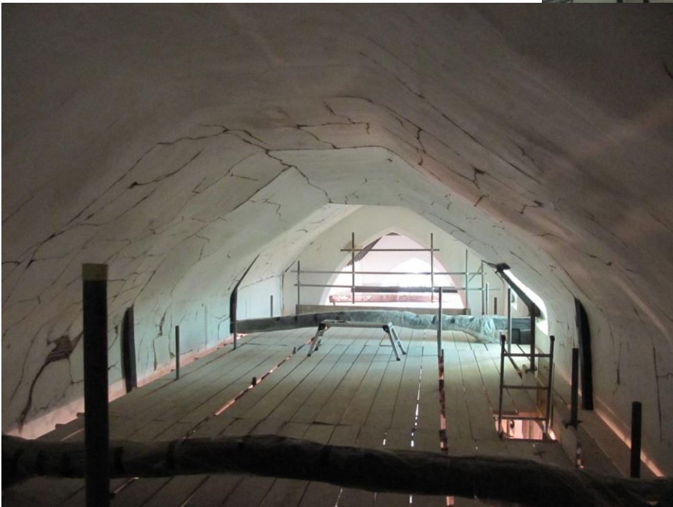
[Church of All Saints Grafham. Nave Ceiling, with views looking east and south]
